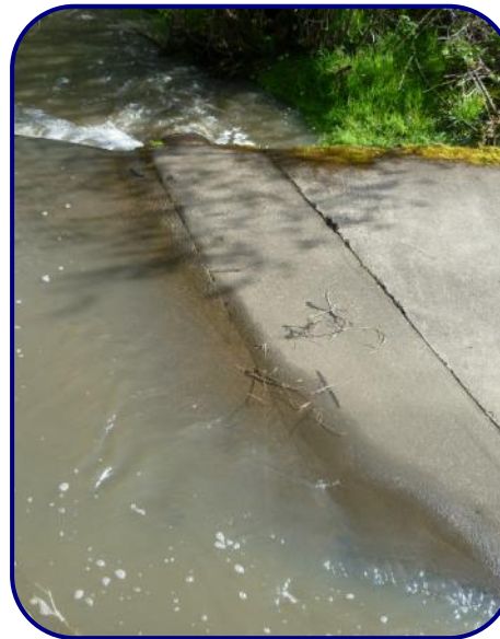
At high flow, this culvert is not large enough to contain the creek.
