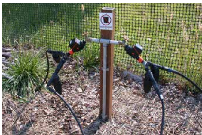
Irrigation system with filters. 14
