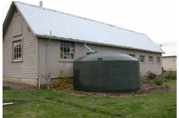
Rainwater harvest tank at OSU's Oak Creek Center for Urban Horticulture. 14
