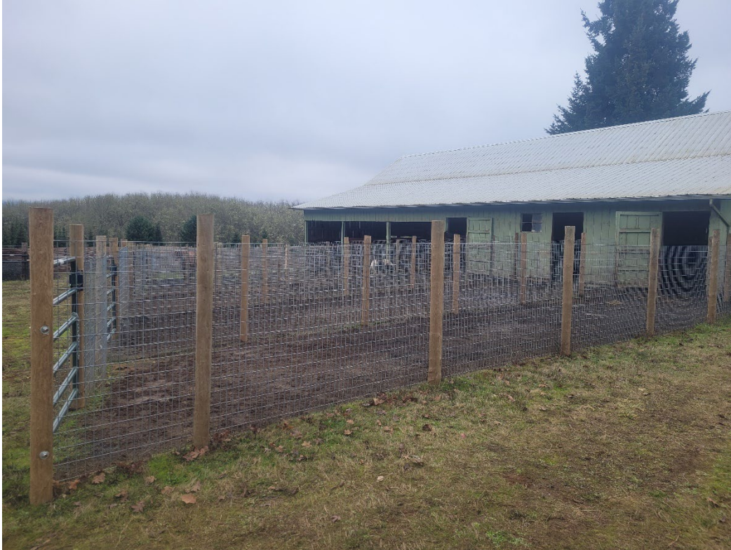
Hawley Creek: Additional hard rock and a French drain is needed to reduce mud and manure during the winter.
