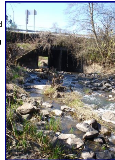
The new culvert allows more fish to access Oak Creek for summer refuge.
