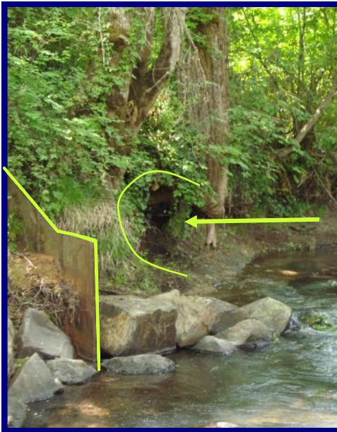
Oak Creek at Urban Hort. Center Note the remnant of dam and severely undercut bank.
